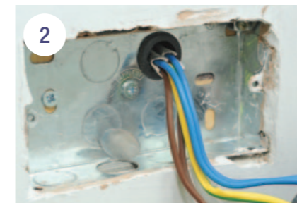
Wood behind the switch box
