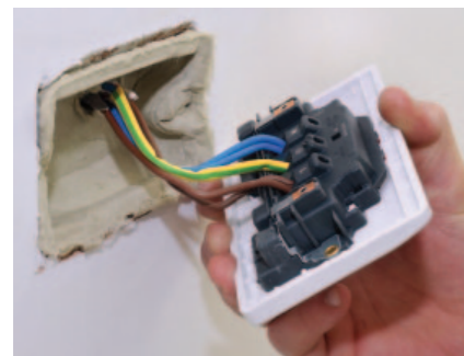
This power outlet in a party wall has an 'intumescent' seal that expands to block the opening in the event of fire
