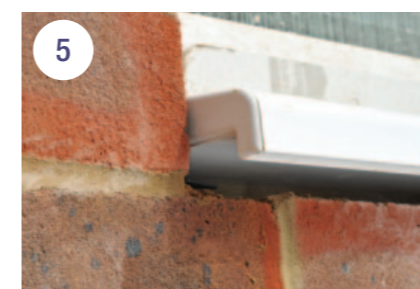
Movement gap under window
